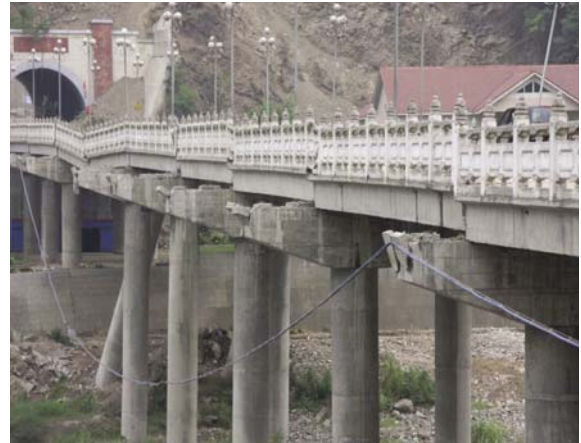
Fig. 16 Damage to a bridge, including a falling deck at the center, at a town in Beichuan County
