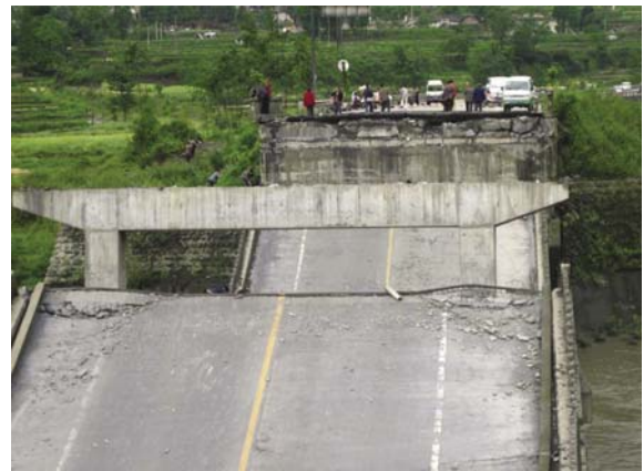
Fig. 17 Xiaoyudong Bridge, two spans near one of the abutments fell down
