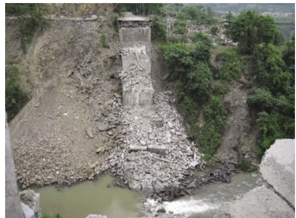
Fig. 18 A totally collapsed bridge, the only access from Hongbai Town to the mountain area from the Shifang City
