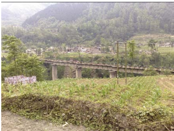
Fig. 15 A severely damaged railway bridge near Yinghua Town, Shifang City
